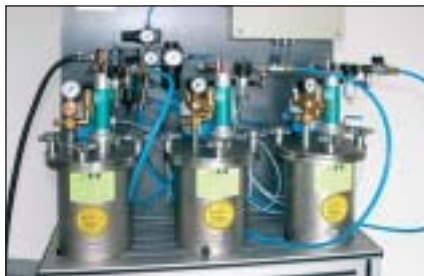
Material supply from pressure tanks for three marking guns
